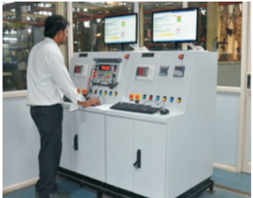
SCADA Test Facility
