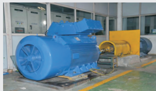
Large Motor Test Facility
